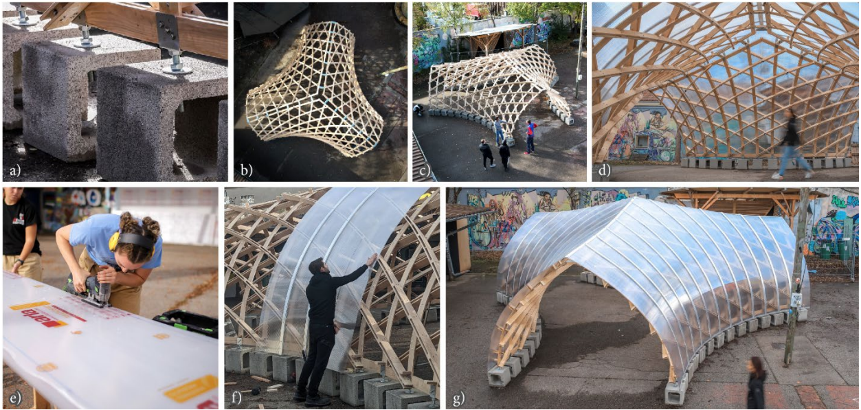
Fig. 9: Completed timber gridshell. Top Row: a) Precast concrete blocks with steel supports. b,c) Birds-eye view of the timber gridshell without cover. d) Inside the Timber Vault. Bottom Row: Polycarbonate panels are tailored with concave edge (e), and installed using aluminum mullions along the geodesic directions (f), to create a smooth, transparent skin (g).
